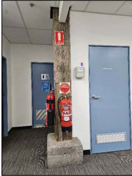
Figure 22. Internal view of original storey post on Ground Floor of subject building, facing south.
