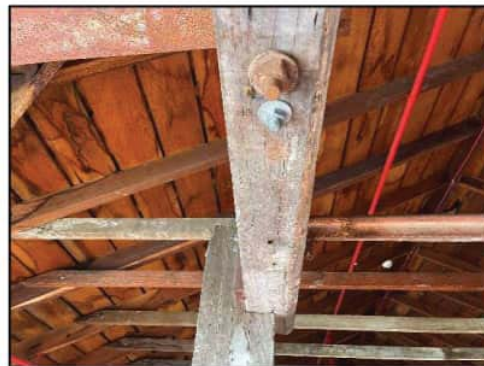
Figure 31. Internal view to the timber roof structure and framing, featuring different bolts (one square head; one hexagonal head).
