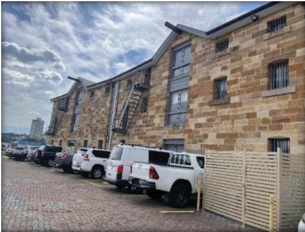
Figure 3: External view of the western elevation of the Moore's Wharf Building, facing north-east (Source: SoHI, October 2024).
