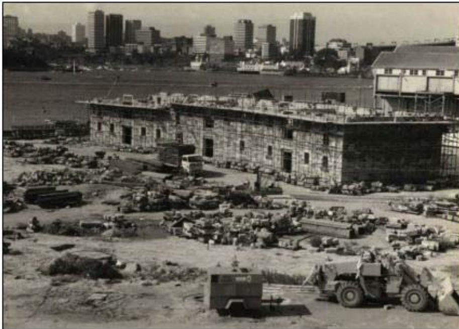
Figure 6-3 The site during reconstruction in circa 1980 (Source: R.J. Lampert & M.C. Truscott in Heritage 21, 2024)
