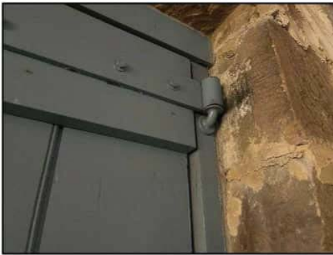
Figure 28. Internal view to the details of a timber door on the Second Floor.
