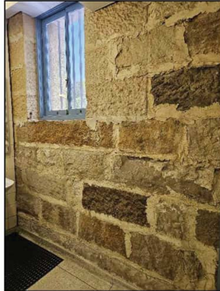
Figure 23. Internal view of original sandstone masonry on Ground Floor of subject building, facing south.
