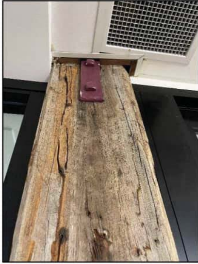
Figure 26. Internal view to a timber storey post on the First Floor, which is experiencing splitting.
