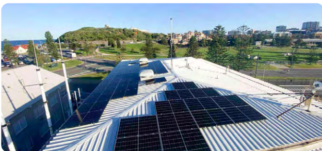
NEW ROOFTOP SOLAR SYSTEM IN NEWCASTLE
