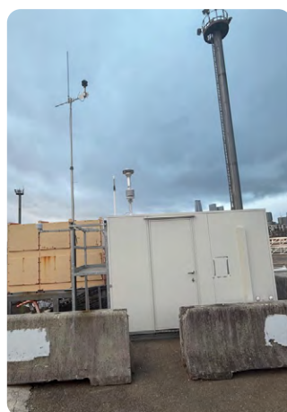
GLEBE ISLAND AIR QUALITY MONITORING STATION
