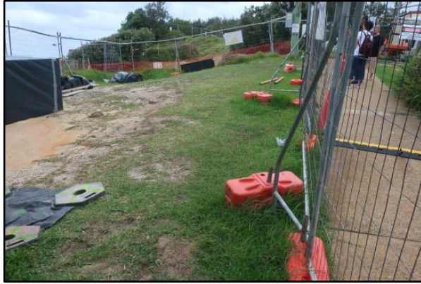
Figure 12. Section of study site south of Hornby Lighthouse, facing south (Source. AMAC Group, 4 March 2024)
