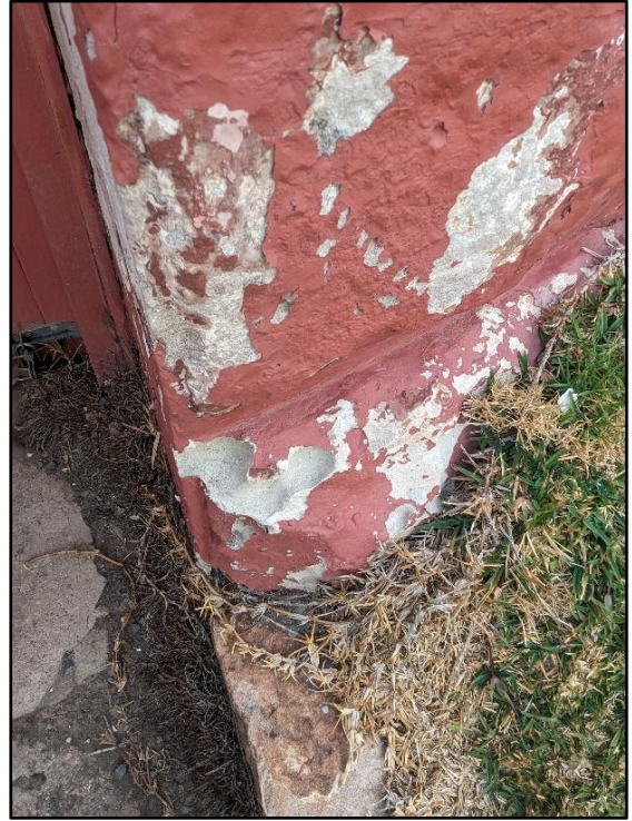
Figure 9. View to damage on the base course of the lighthouse, due to water and soluble salt ingress (prior to the conservation works).
