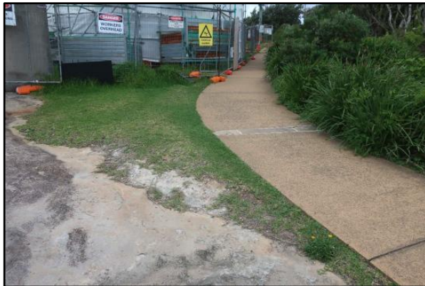
Figure 10. Section of study site north of Hornby Lighthouse, showing small amounts of fill on bedrock, facing south (Source. AMAC Group, 4 March 2024)
