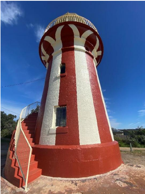
Figure 2-4 External view to the lighthouse, at the completion of the conservation works in August 2024 (source: SOHI, Heritage21, 2025).
