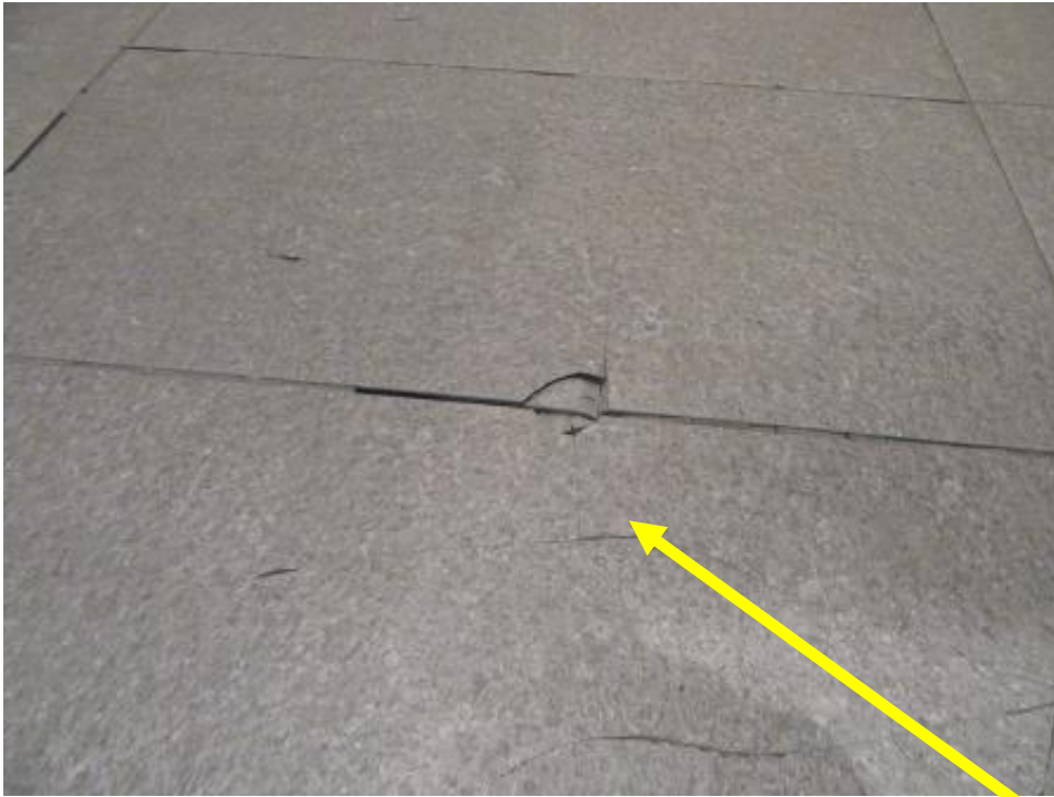
Lift 9 – the lift car floor tiles are damaged and need to be replaced
