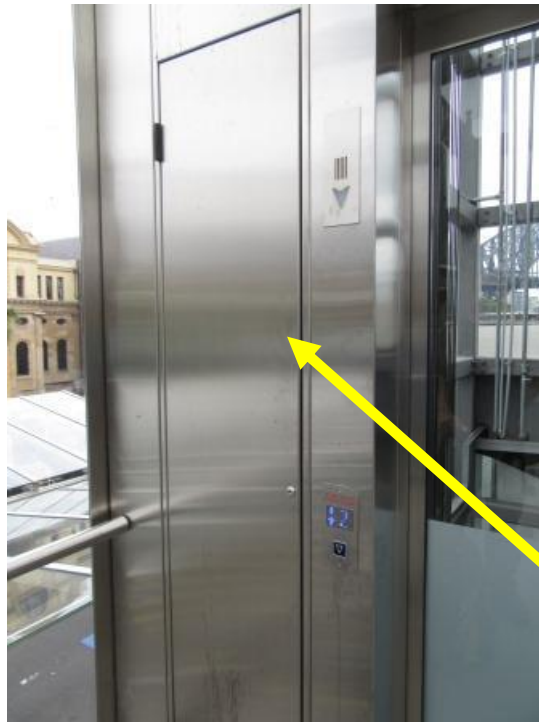
Lifts 7-10. Regulation electrical warning notices are required on the lift controller doors
