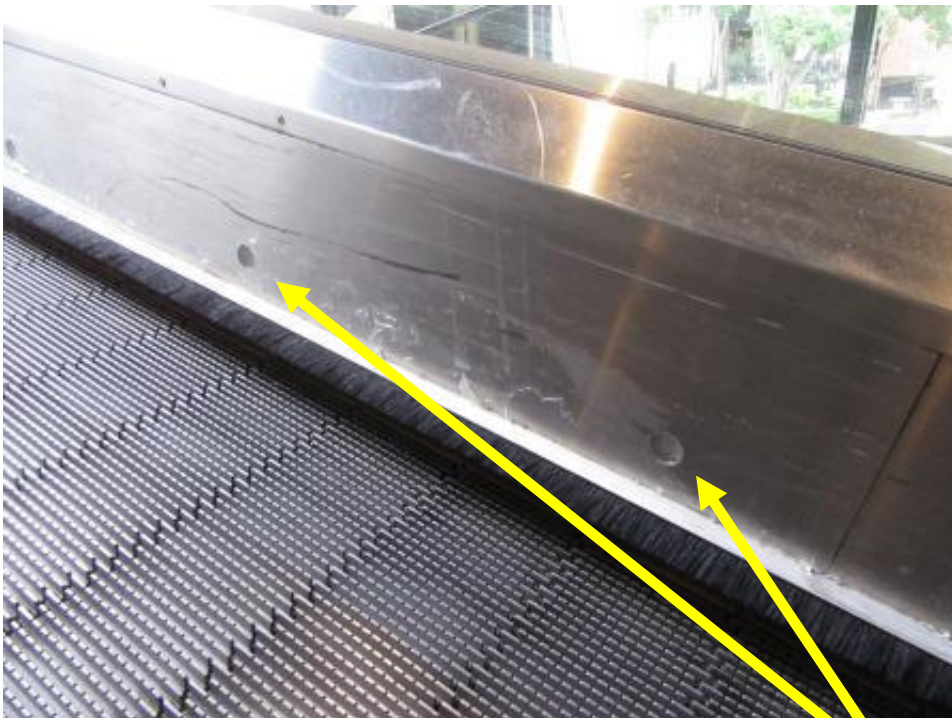
The skirting lighting on the moving walks is inoperative
