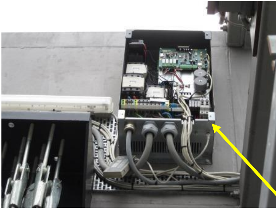
The VVVF drive units and emergency evacuation units on lifts 7-10 are virtually inaccessible and should be relocated
