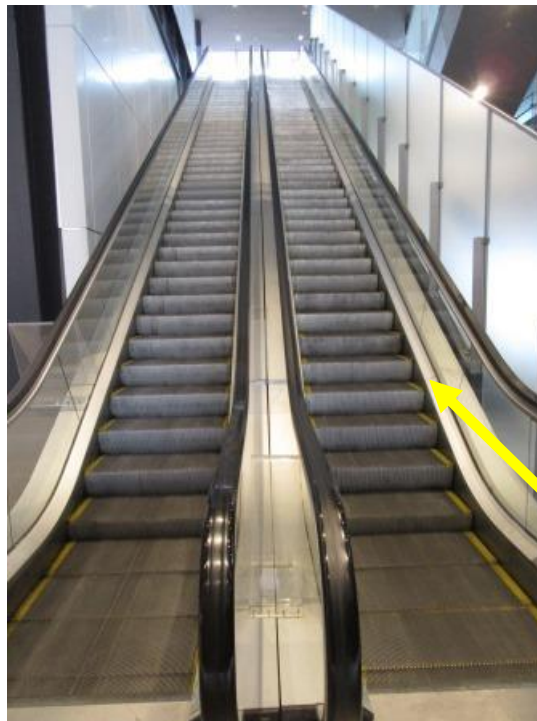
Escalators 1 & 2 were relocated from outside the main building to inside it around 9 years ago. These units are now around 30 years old.
